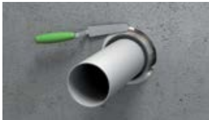
5. Ensure smoke tight seal of the annular gap. Seal it with a gap filler like Walraven Pacifyre® A acrylic sealant, Pacifyre® H hybrid sealant (fill depth = 10 mm) or Walraven Pacifyre® FPM fire protection mortar.
