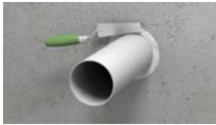
2. Close the gap with loose mineral wool and seal it with a gap filler like Walraven Pacifyre® A acrylic sealant, Pacifyre® H hybrid sealant or Walraven Pacifyre® FPM fire protection mortar (fill depth = 10 mm).
