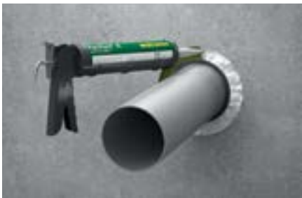
4. Ensure smoke tight seal of the annular gap. Seal it with a gap filler like Walraven Pacifyre® A acrylic sealant or Walraven Pacifyre® FPM fire protection mortar (fill depth = 10 mm).
