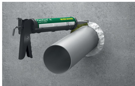
2. Close the gap with loose mineral wool and seal it with Walraven Pacifyre® A Acrylic Sealant (fill depth = 10 mm).
